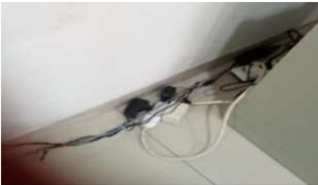
Figure 6: The electrical line connection.
